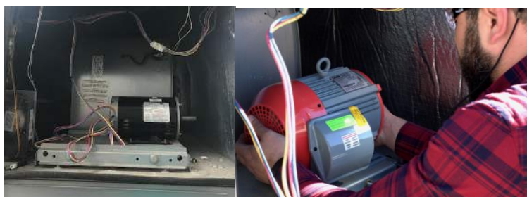
Figure 1. (Left) Legacy motor and (right) SMC motor installed in a 10-ton RTU.
